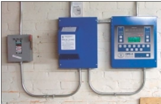
The Tjernlund System controls include VFD in the middle and CPC-3 Constant Pressure Controller on right
