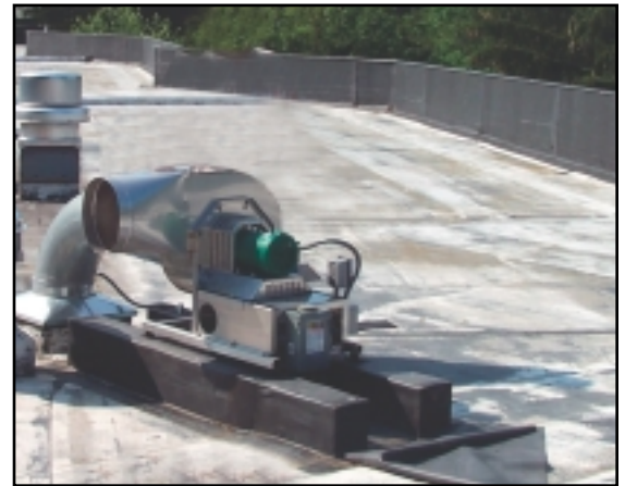
Roof-mounted Tjernlund VSUB fans (above) were selected to exhaust dryers because they modulate to save energy and are easy to clean.
