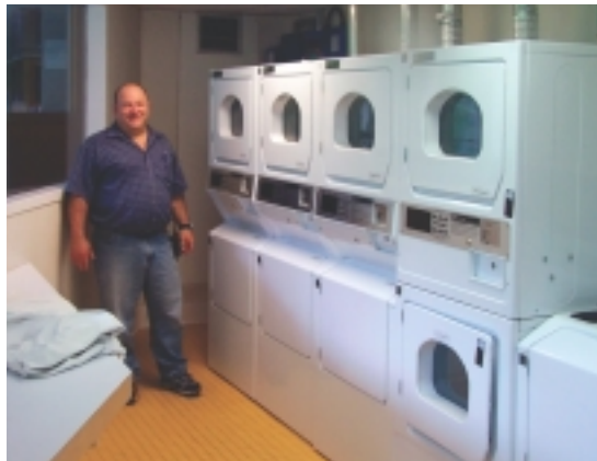
Ken Jensen of Williams College said energy savings from revised dryer vent system was in step with the school's goal of reduced energy consumption.
